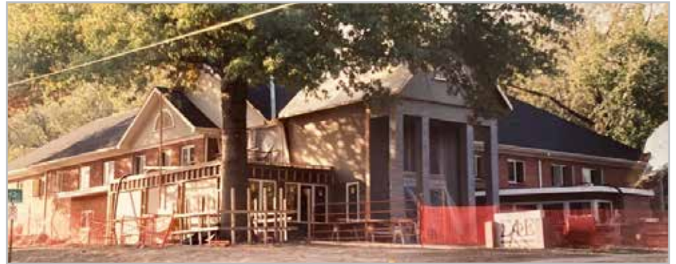
1991 | 1645 Tennessee Street. Post fire & first major expansion with addition of new entryway, library and Presidential Suite.
